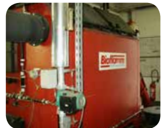
Sainte-Marie-aux-Mines – Chaufferie bois © Energivie
